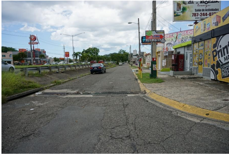
Photo 19: Street intersection with patched up pavement and storm-water drain catch
